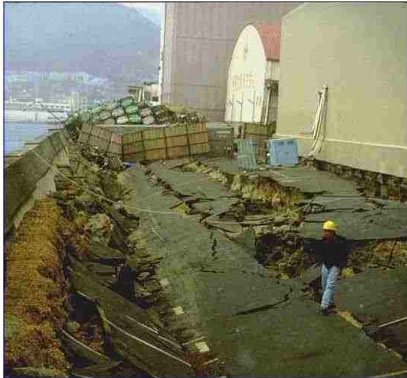
Figure 5.2. Liquefaction-induced lateral spreading from the 1995 Kobe, Japan earthquake causing severe damage to a quay wall (UW).
