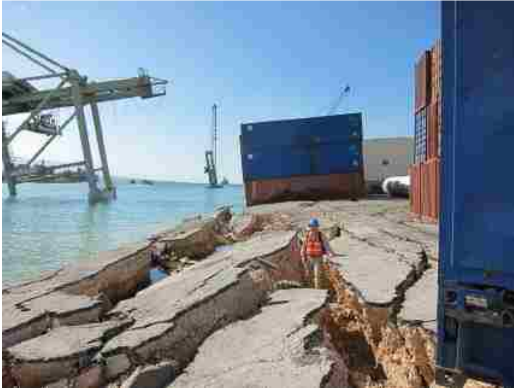
Figure 2.2. Liquefaction-induced lateral spreading at the North Wharf of the Port de Port-au-Prince (photo from DesRoches et al., 2011).
